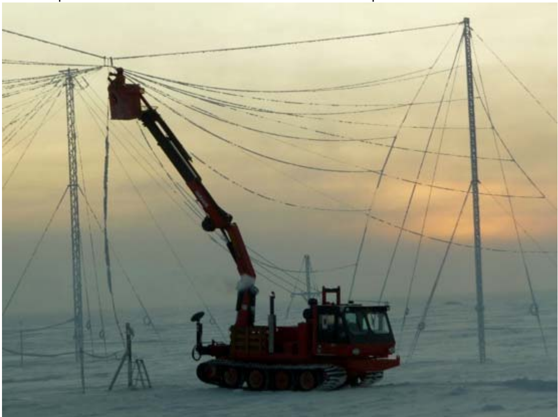
Photo 4: Me doing part of my daily maintenance tasks. Fixing the North-South HF antenna which snapped due to the extreme cold
